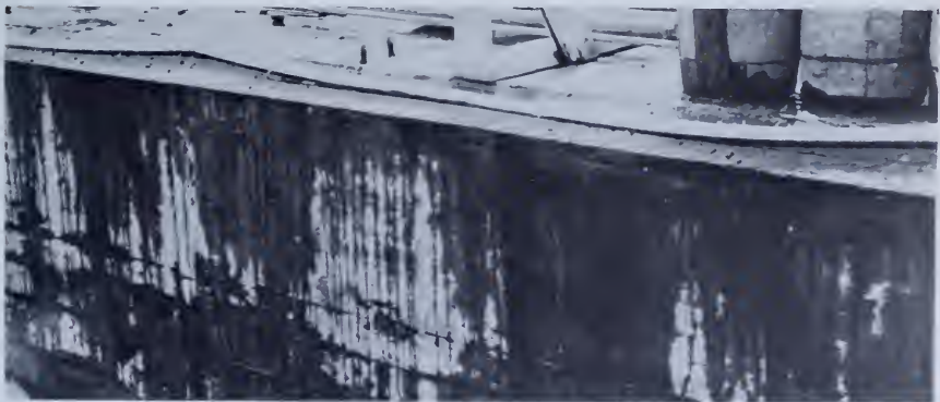
Figure 172.—Water curing with soil-soaker hose. This prevents rust stains which may occur if iron pipe is used. PX-D-34609.
